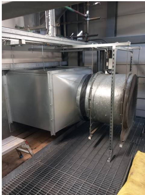
Figure 1-3 Turbine Hall Works as Installed
