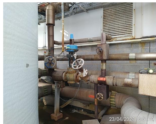
Figure 7. Steam return valve 10BLB10GH010, behind polished water storage tank 1
