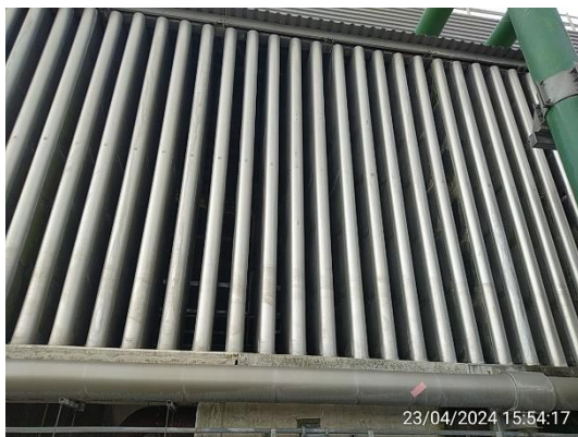
Figure 5. Silencer baffles in front of Phase I cooling tower air inlet
