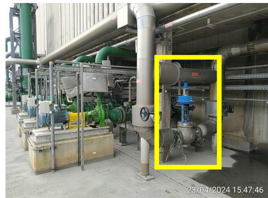
Figure 9. Valve 10PAR10AA001X (yellow box)
