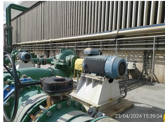
Figure 8. Phase I water pumps overview
